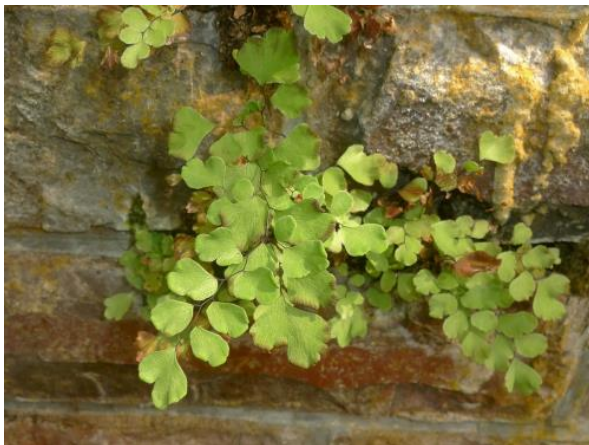
Fig. 9: Adiantum capillus-veneris . Small plants growing from cracks in a brick wall.
